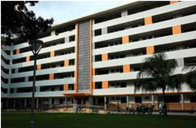
Fig 2: Common corridor along the building facade having laundry being exposed and dried along the common corridor and window openings.
